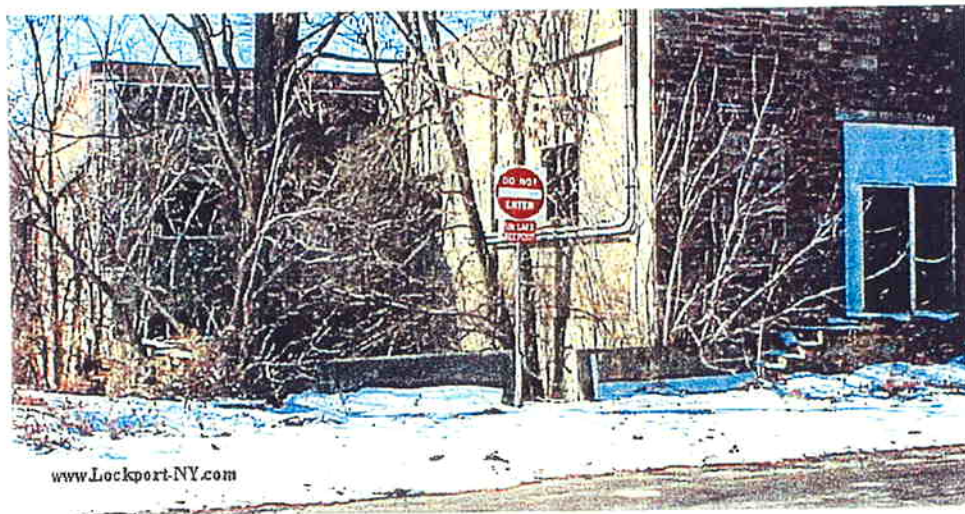
Figure 6-2. Photograph of the former Flintkote buildings at Mill and William Streets looking west. These buildings have been abandoned for many years and are extremely dilapidated. The concrete barriers prevent vehicle traffic from entering William Street, which passes under the building in the background. Photo from www.Lockport-NY.com
