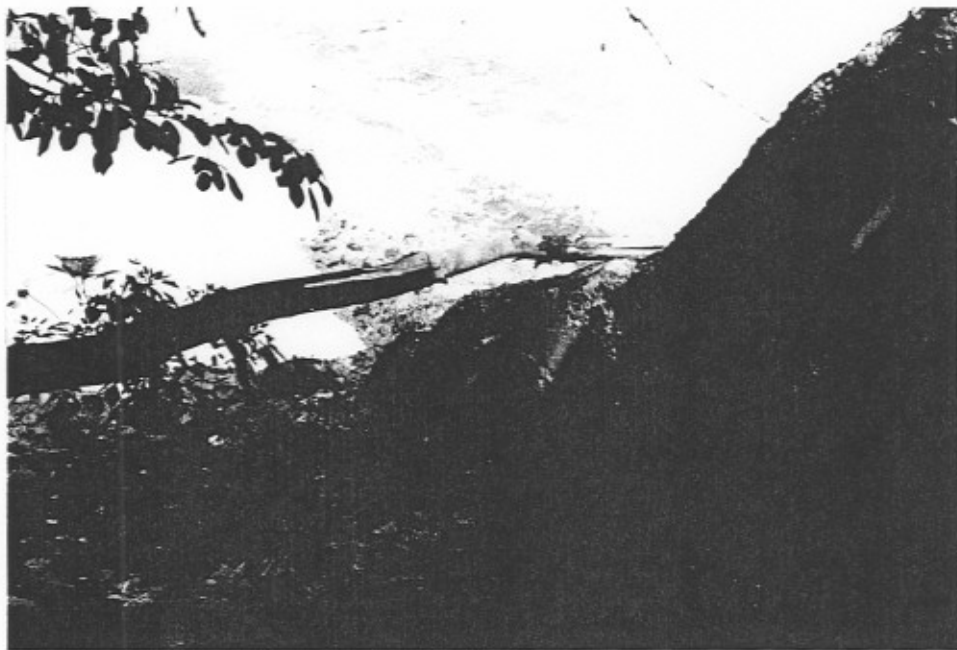
12. West face of west spillway wall. Note spalled concrete.
