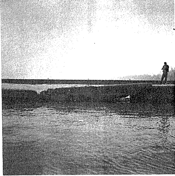
Photo No. 5 - View from lake side of section of pier from Sta. 4+50 to 4+90. Note east pier, repaired in 1949, in background of this and Photo No. 4.
