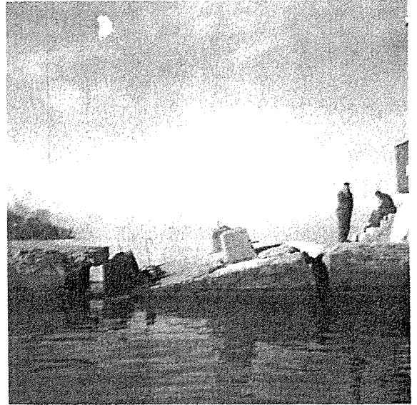
Photo No. 2 - View from channel of section of pier from sta. 2+35 to 3+15.
