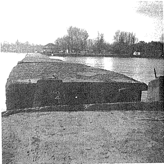
Photo No. 3 - View along pier crest toward shore from steps shown in Photo No. 1. Shoreward sections of crest show evidence of differential tilting of timber crib substructure.
