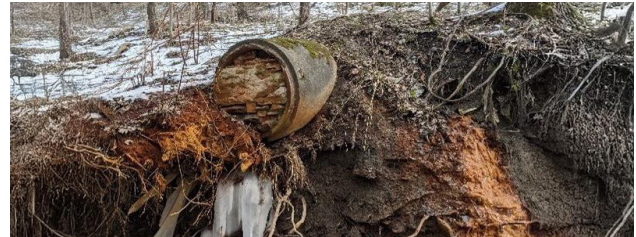
Pre-remediation Lockport City Landfill seep
