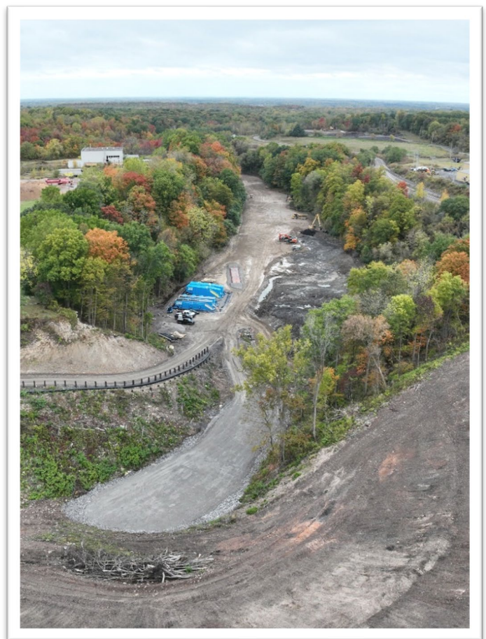
Drone imagery of the progress former dump site excavation (foreground) and Gulf Creek sediment excavation and backfilling, October 2023.
